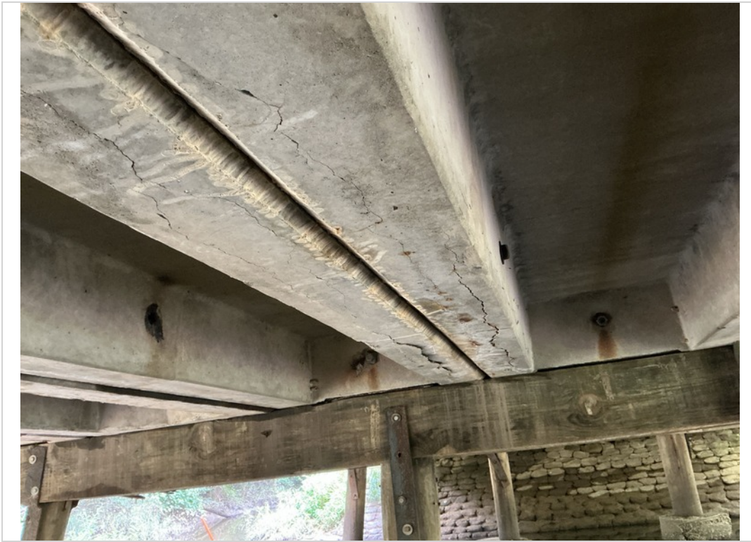
Span 3 Beams D & E Delaminations
