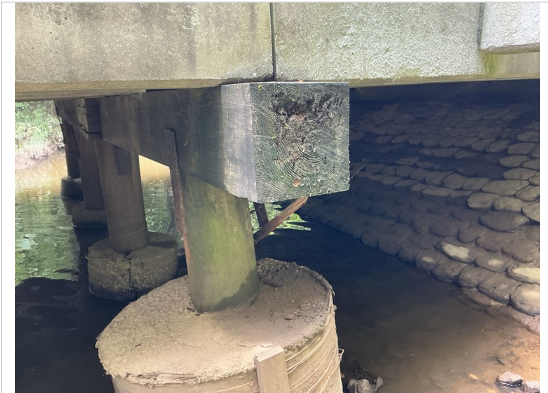
Bent 1 Cap LT Minor Decay/Weathering
