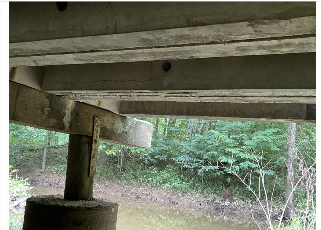
Span 3 Beam B Delamination
