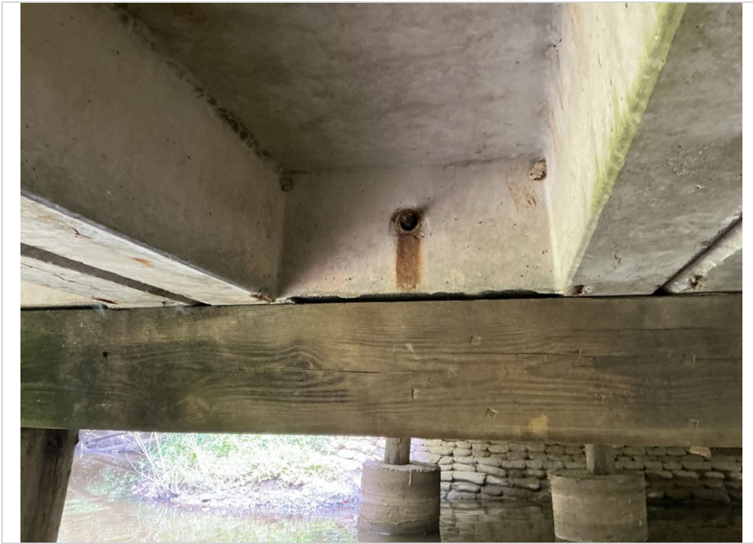
PCCS Missing Bolts Typical
