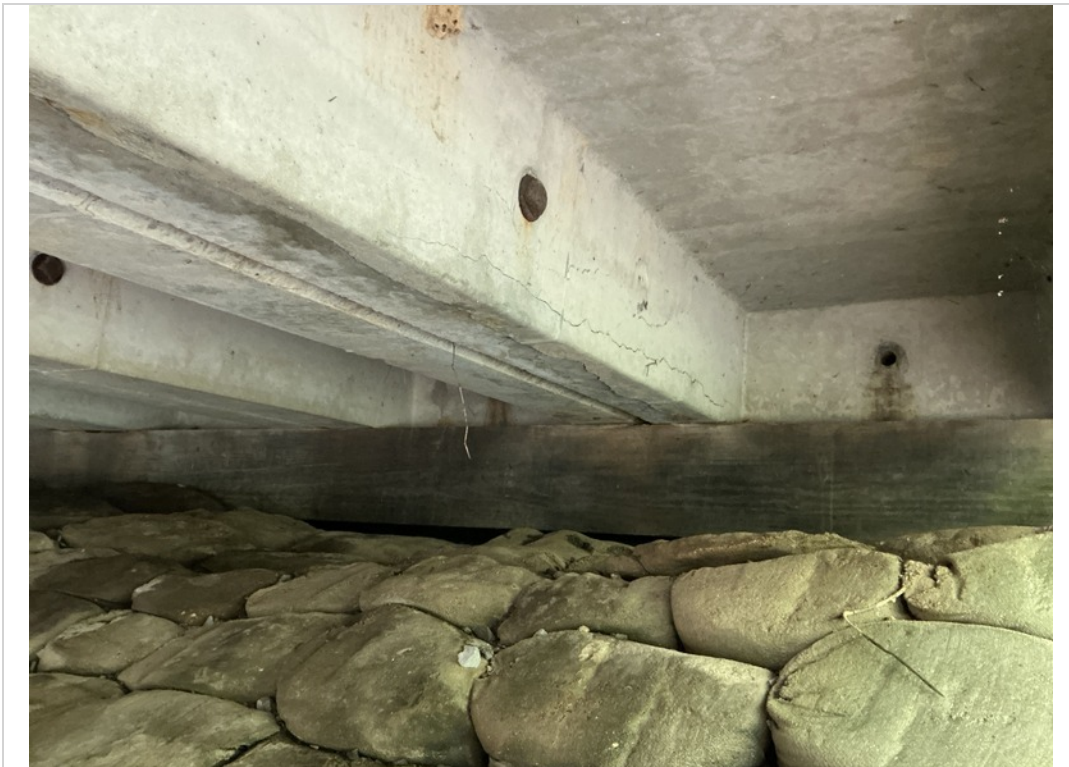
Span 1 Beam A Delamination
