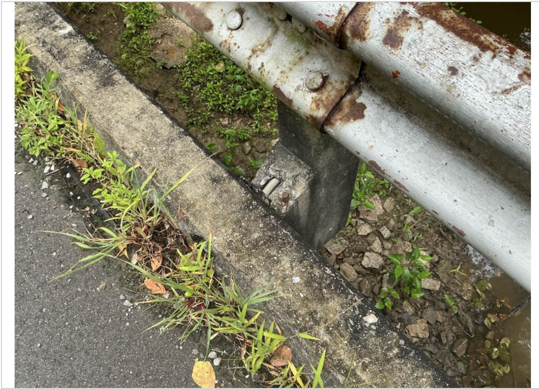
Concrete Rail Post Spalls at Anchor Typical
