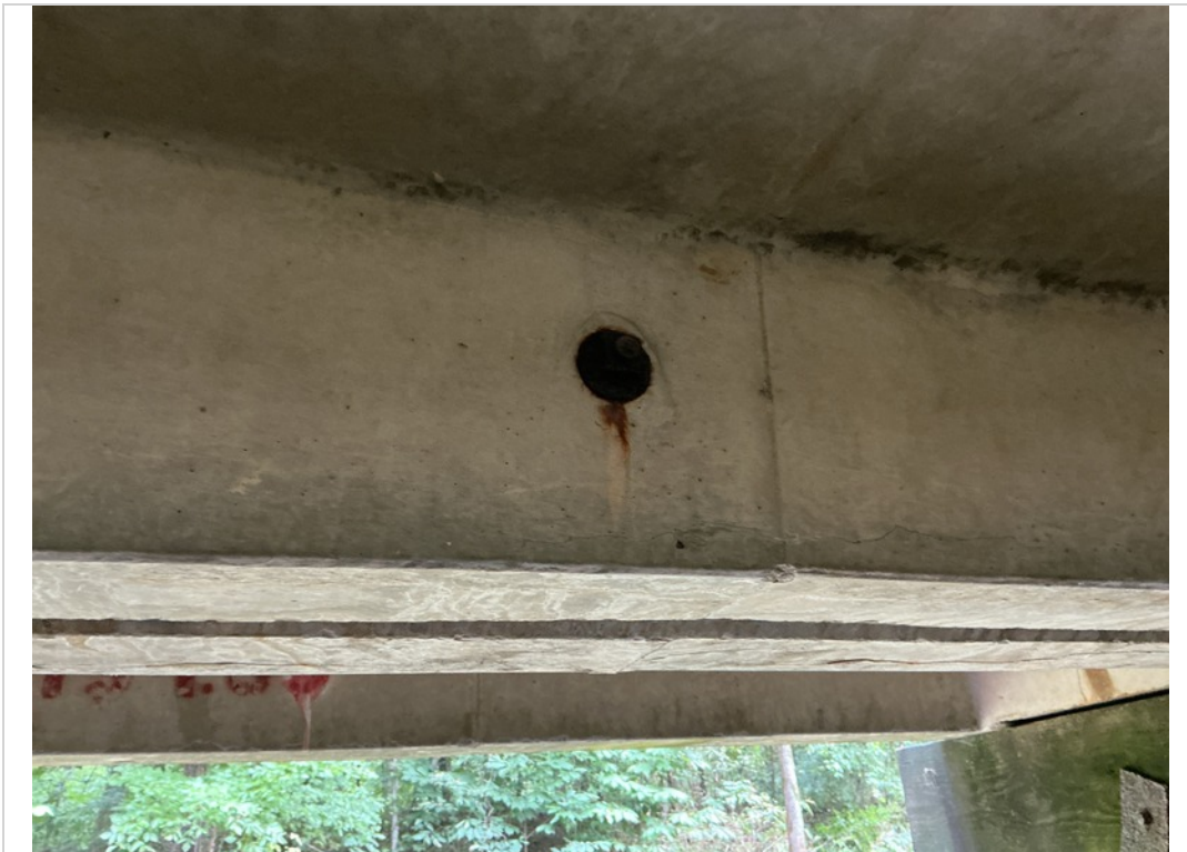
PCCS Bolt Corrosion Typical
