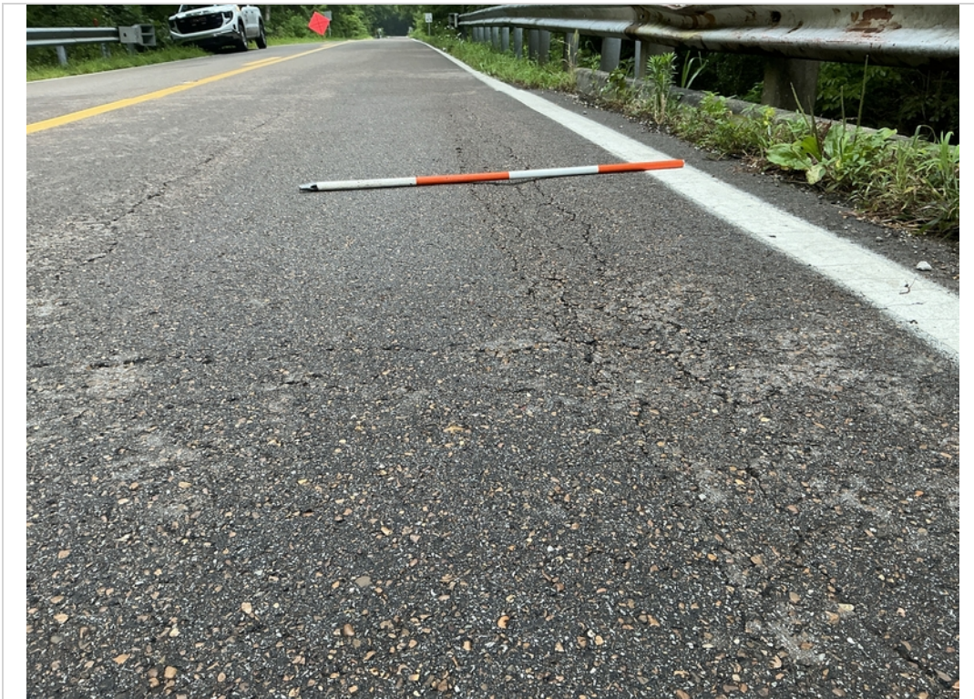
Spans 2 & 3 Settlement Between Beam Edges
