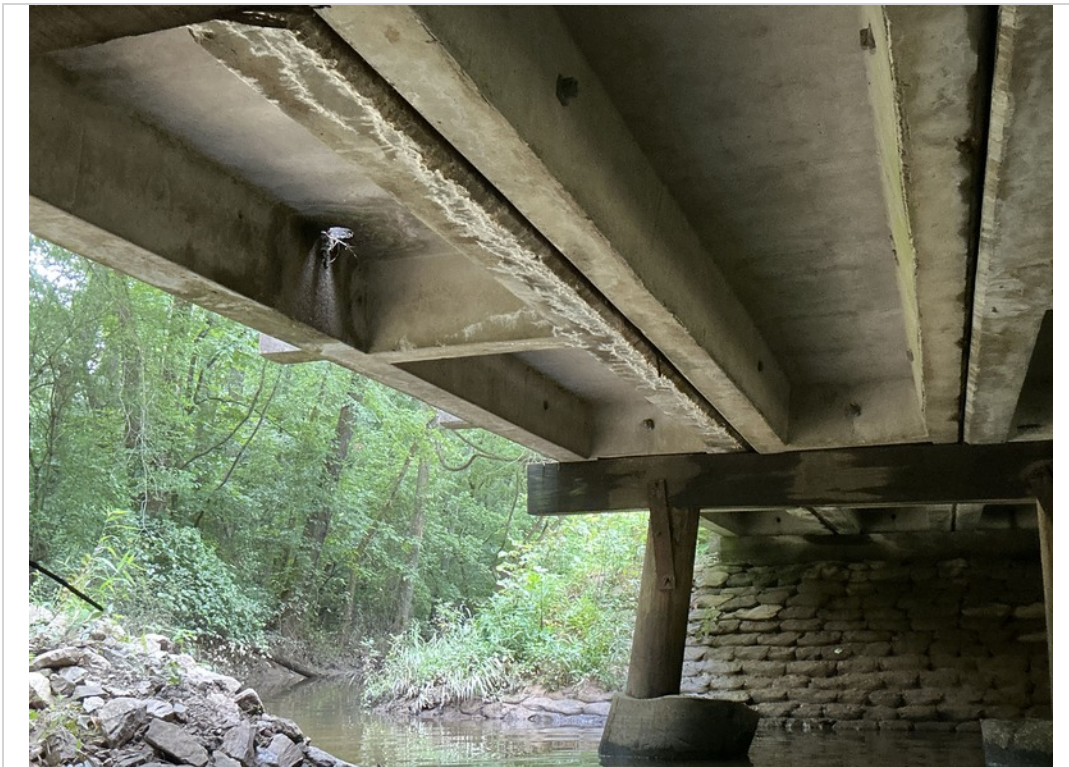
Span 2 Beam G Hairline Cracks w/EFF
