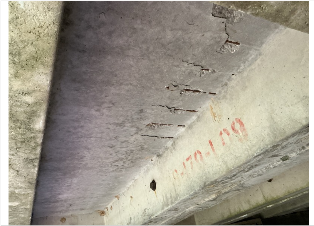
Span 1 Beam A Cover Spalls in Soffit
