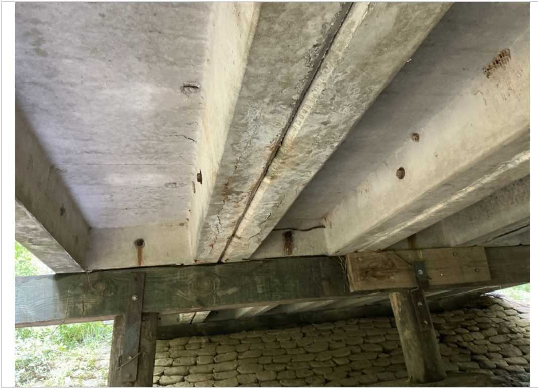
Span 2 Beams A & B Delamination
