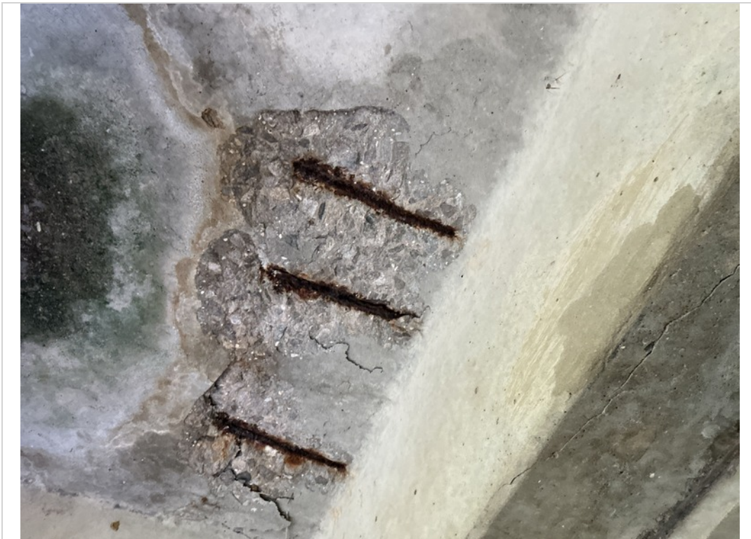
Span 2 Beam A Cover Spalls in Soffit
