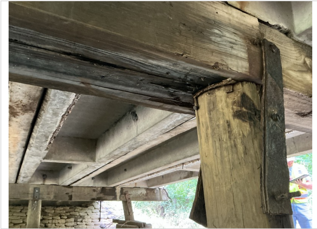
Bent 1 at Pile C Minor Decay, Splitting/Shake at Cap Section End at Bearing Point
