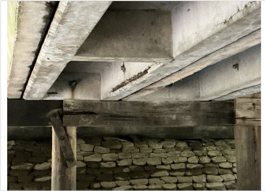
Span 2 Beam E Spall w/Exposed Rebar
