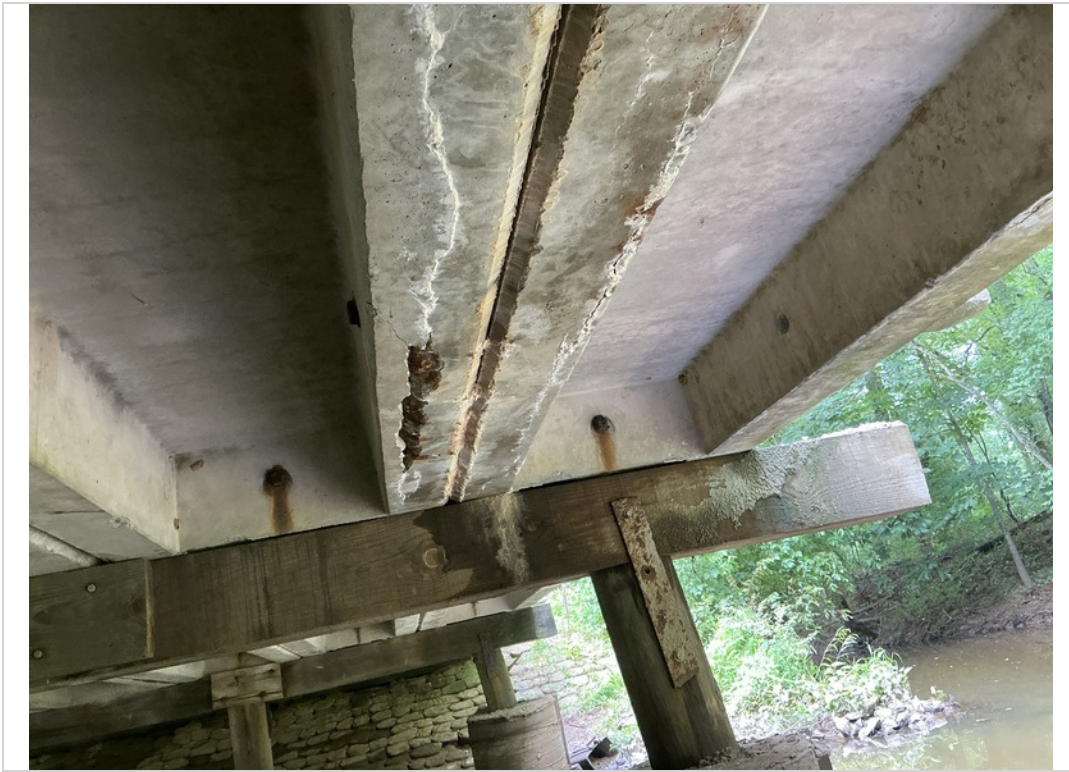
Span 3 Beam B spall and Hairline Cracks w/EFF
