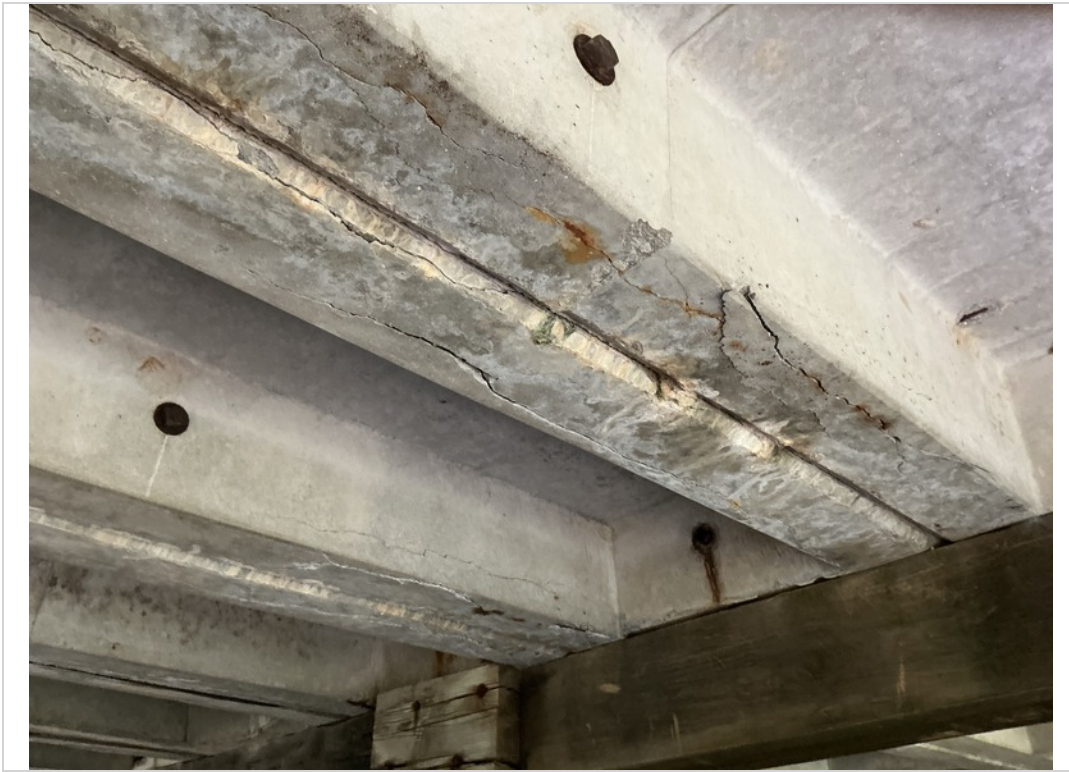
Span 2 Beams A & B Delamination
