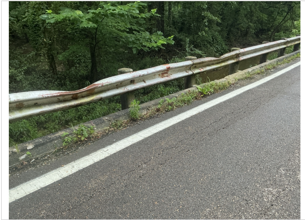
RT Rail Minor Impact Damage
