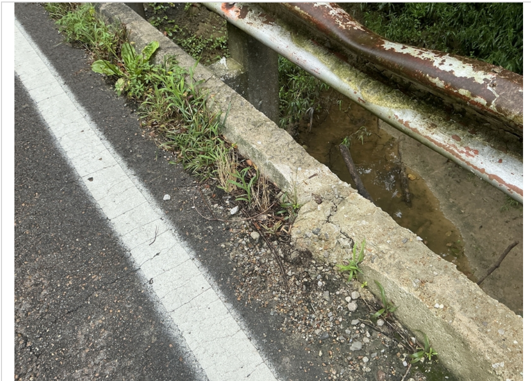
Span 2/3 RT Curb Spall with exposed Rebar
