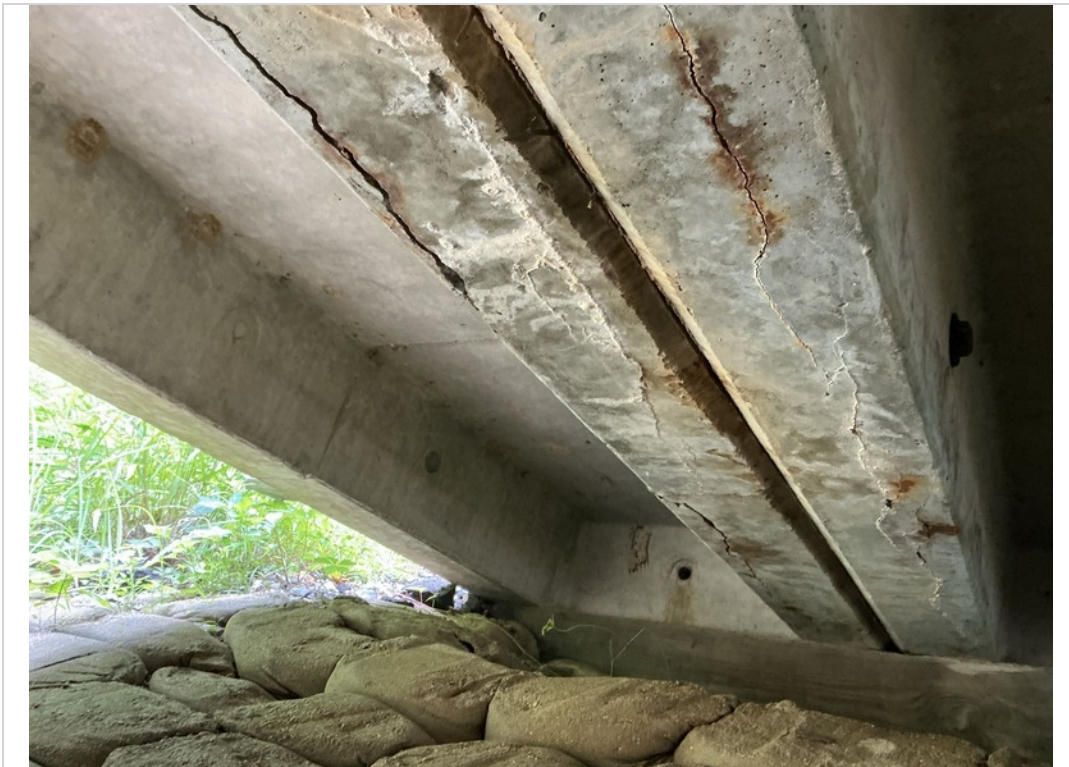
Span 3 Beams A & B Hairline Cracks w/EFF
