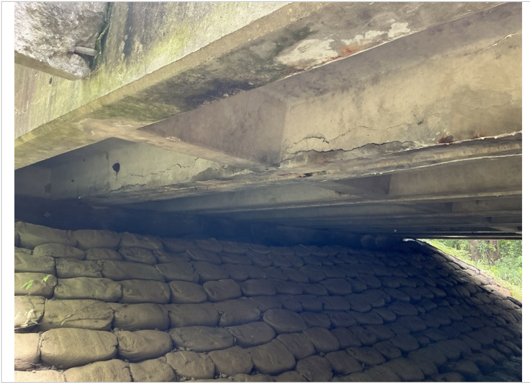
Span 3 Beam A Delamination
